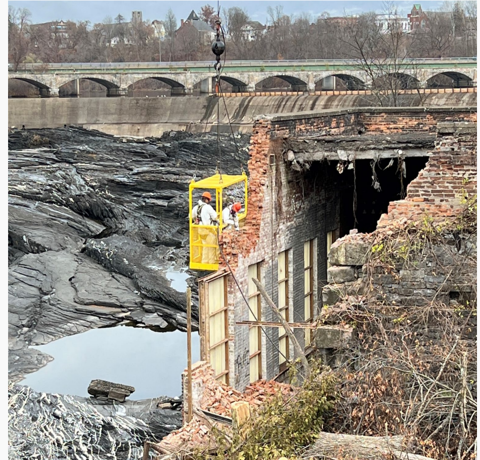
This photo shows the Powerhouse building being carefully dismantled using hand tools to limit disturbances to bedrock and minimize fallen debris into the river
